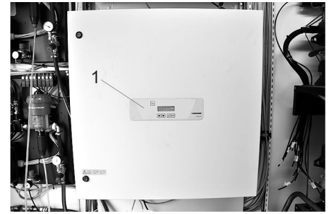
1 Fault indicator in the display of the control
