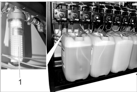
1 Filter for frost-protection pump
